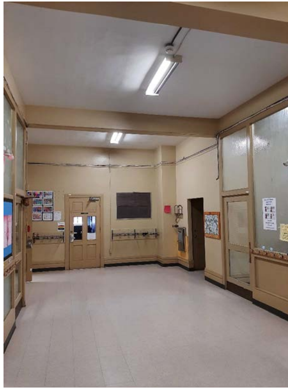
Photograph No. 5 – The beige paint on interior walls is lead-containing.
