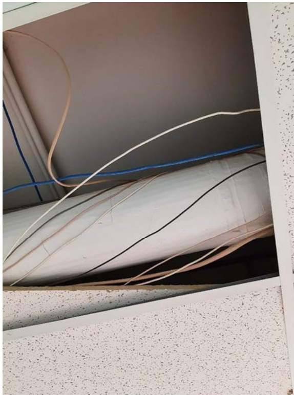
Photograph No. 4 – Asbestos-containing aircell pipe insulation was observed on pipe straights in the basement above ceilings throughout. Associated parging on pipe fittings also contains asbestos.
