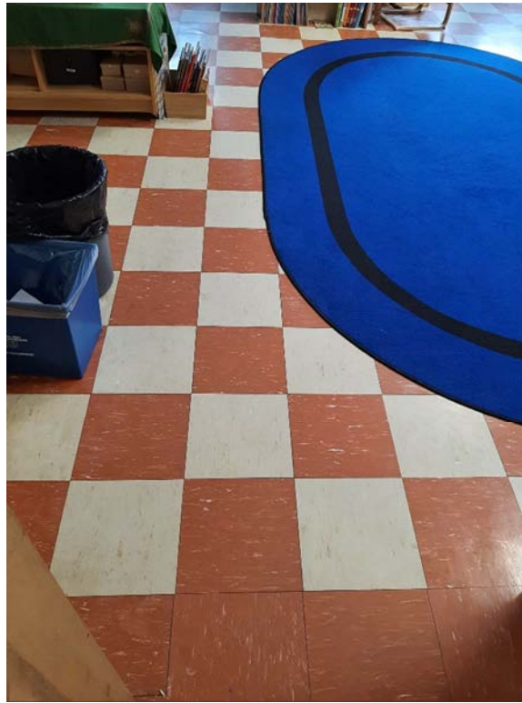
Photograph No. 1 – The Vinyl Floor tile in classrooms 218 and 215 is asbestos-containing. The associated mastic is non-asbestos.
