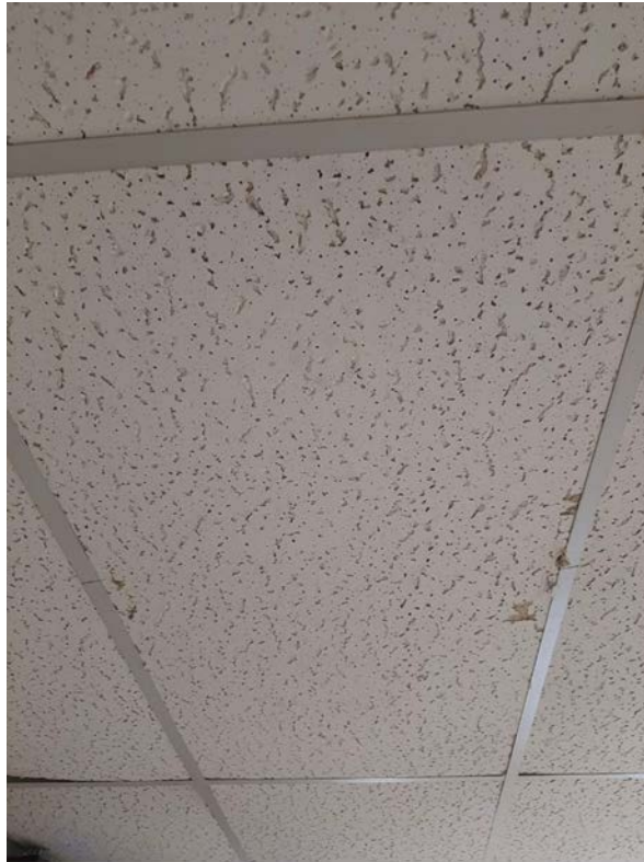
Photograph No. 13 – 2'x4' medium fissure random pinhole ceiling tile was sampled in room 205 and does not contain asbestos.
