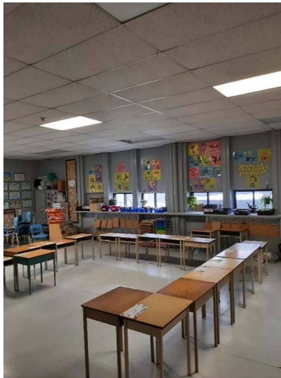
Photograph No. 6 – The grey paint on walls in classrooms is lead-containing.
