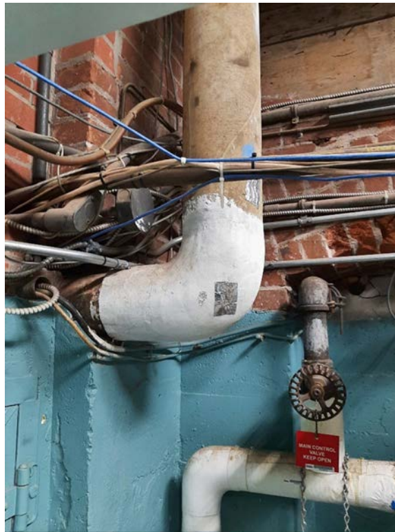
Photograph No. 2 – Aircell pipe insulation on pipe straights throughout the boiler room and adjacent mechanical rooms is asbestos-containing. The parging on pipe fittings is also asbestos-containing.
