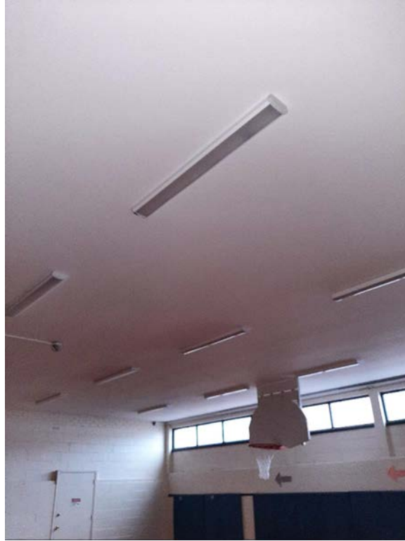
Photograph No. 10 – The drywall ceiling in the Gymnasium does not contain asbestos.
