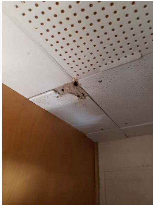
Photograph No. 14 – 1'x1' small pinhole and large pinole ceiling tiles above the drop ceiling in Room 205 were sampled and do not contain asbestos. These same tiles are present at various locations throughout the ground floor.
