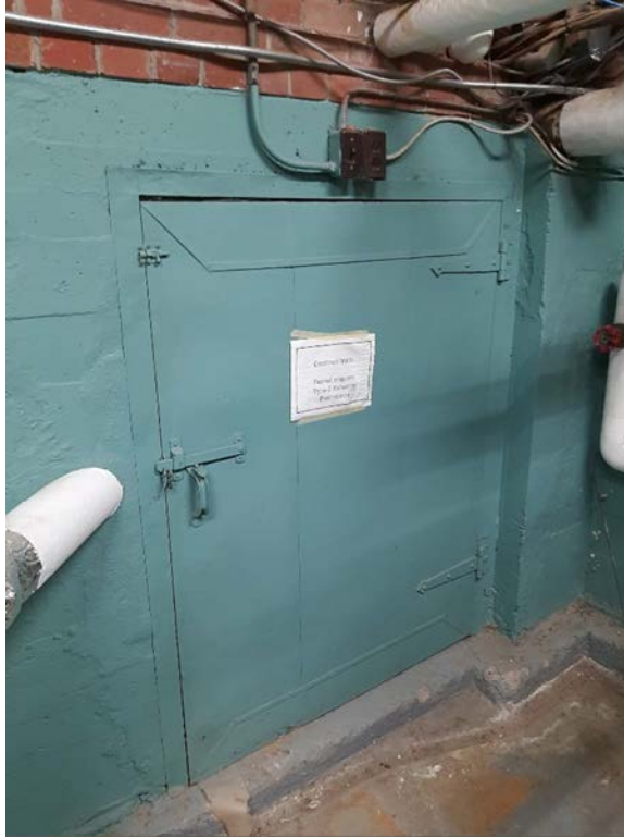
Photograph No. 3 – Fire doors were observed in the boiler room and are suspected to contain asbestos insulation.
