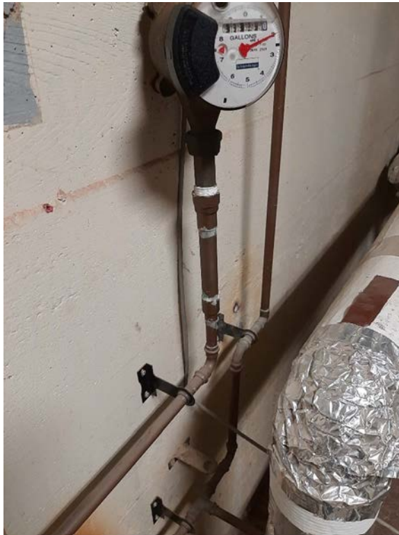
Photograph No. 10 – Suspect lead solder on copper piping was observed in the boiler room.
