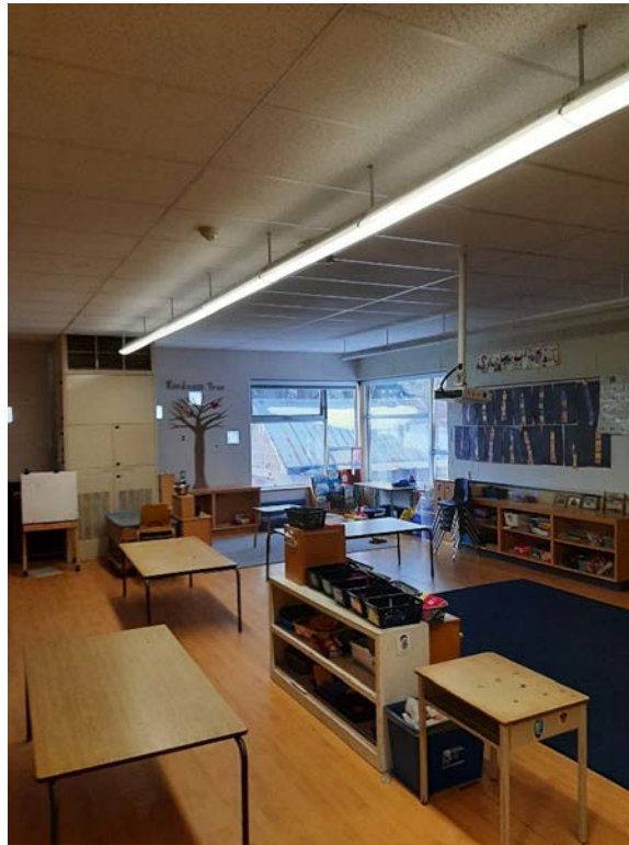
Photograph No. 12 – Mercury contain fluorescent light tubes were observed throughout the interior. Associated light ballasts could not be de-energized and accessed; therefore, they are suspected to contain PCBs.
