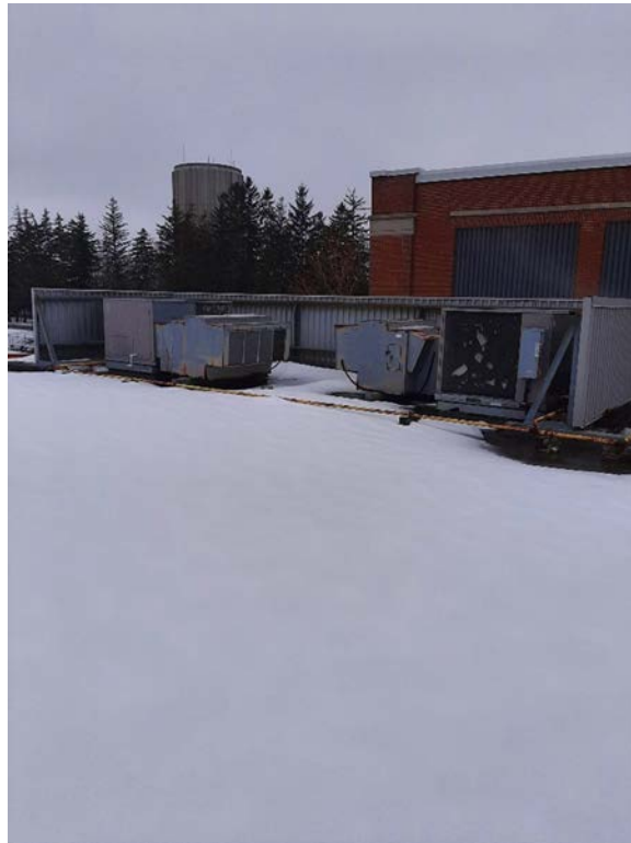
Photograph No. 11 – Roof mounted air handling units were observed and are suspected to contain ozone depleting substances.
