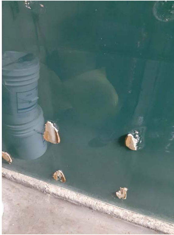
Photograph No. 16 – The mastic behind the classroom chalkboards was sampled and is asbestos-containing.
