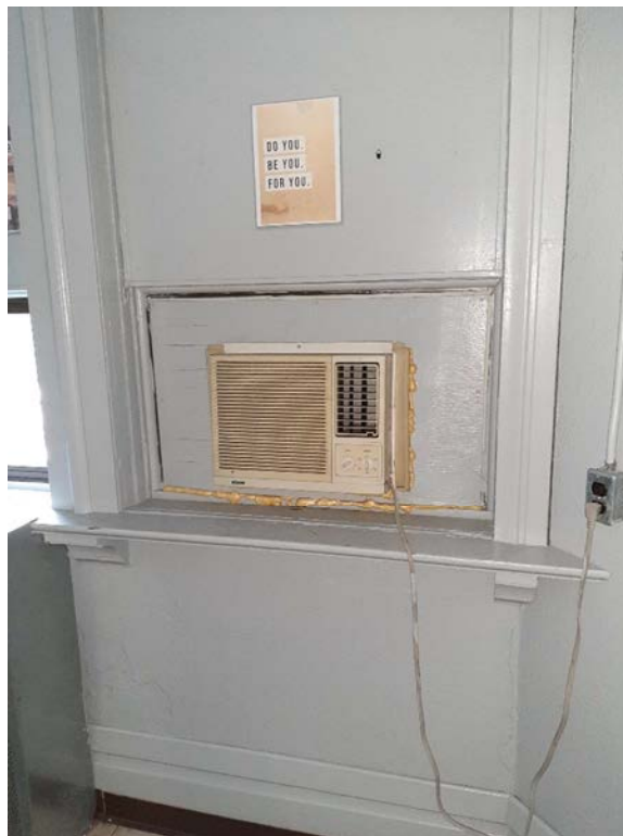
Photograph No. 8 – Window mounted air conditioning units were found throughout the building in classrooms and are suspected to contain ozone depleting substances.
