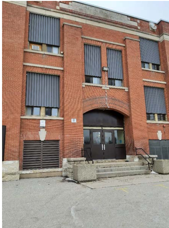
Photograph No. 7 – The white paint on the foundation is lead-based. The brown paint on exterior doors and windows is Lead-based. The exterior brick mortar was sampled and does not contain asbestos.
