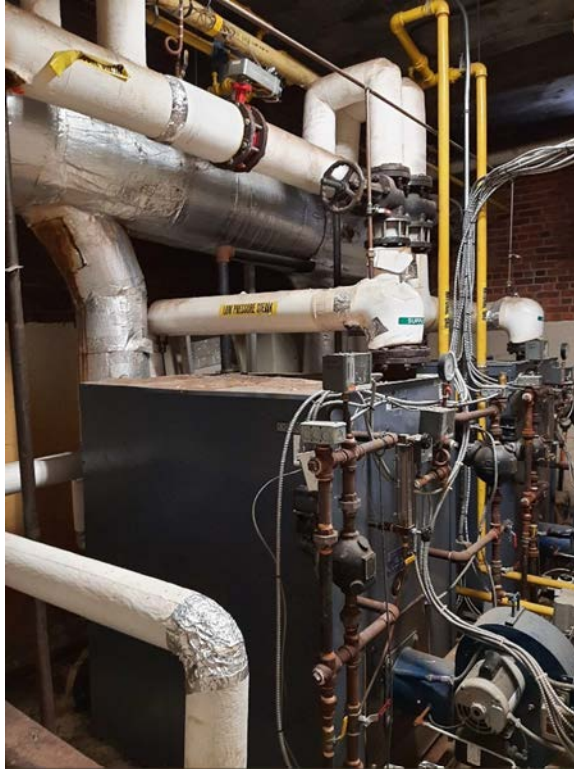
Photograph No. 9 – The boiler is suspected to contain asbestos components such as gaskets.
